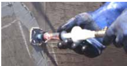
Injection of BL-GROUT with pump and state of BL-INJECTOR during pressurized injection of grout material
